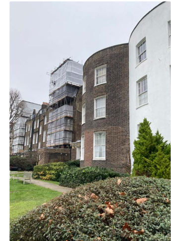
Above: scaffolding at Highbury Terrace where we have now completed major roof repairs.
