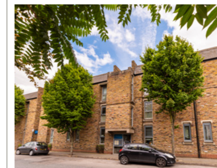
Heavy downpours have caused far more roof leaks this last year
